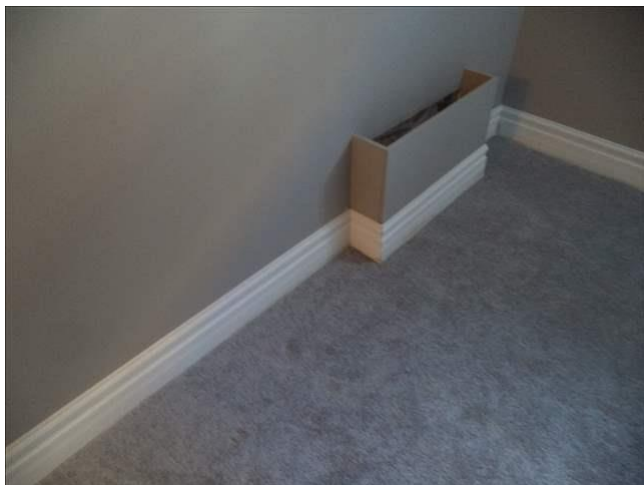
Moisture detected with moisture meter
