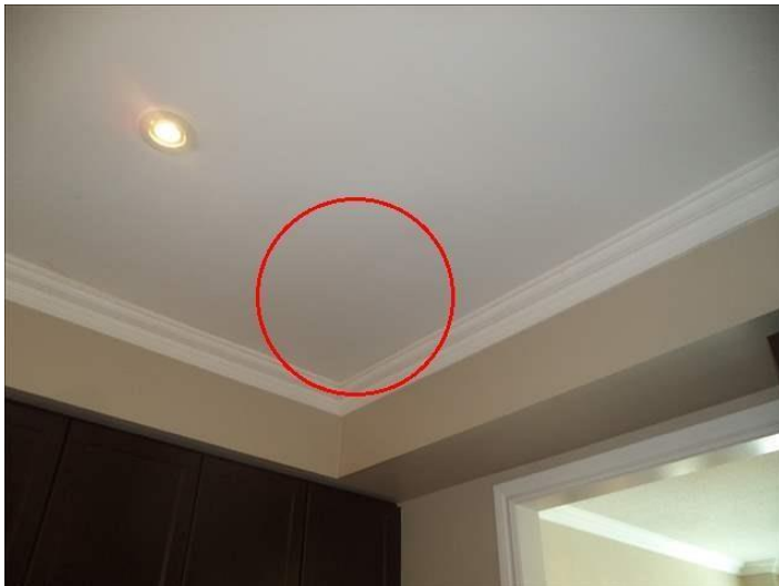
Moisture detected with moisture meter
