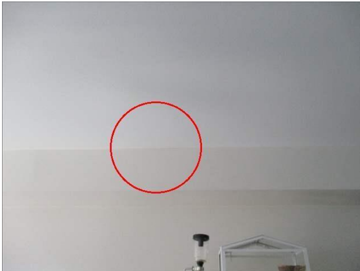
Moisture detected with moisture meter
